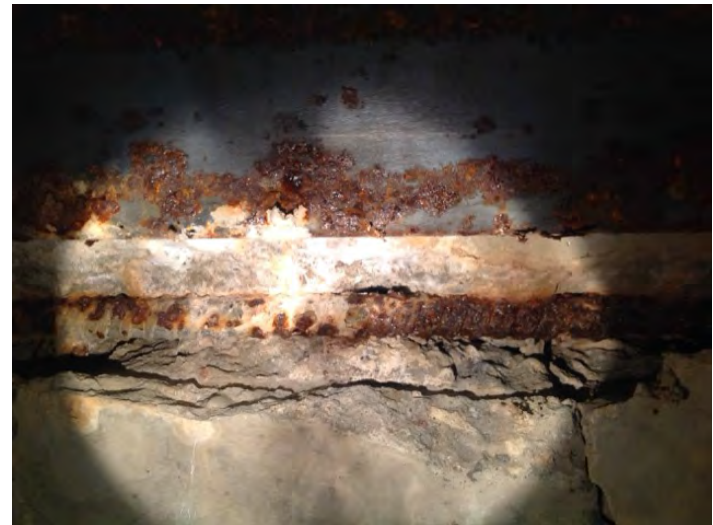
left abutment panel damage
