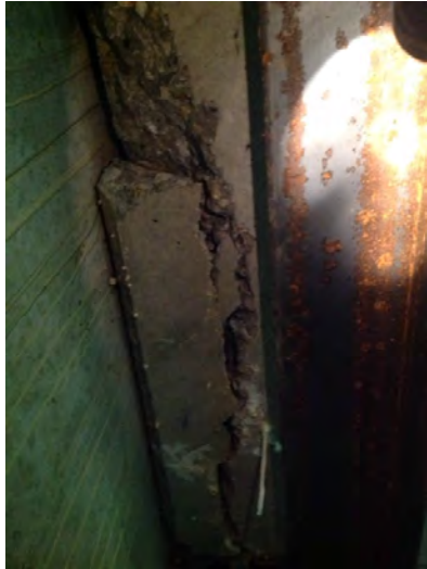
panel 1 on right bank damage
