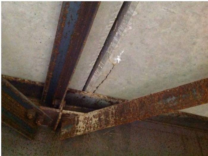
small panel damage
