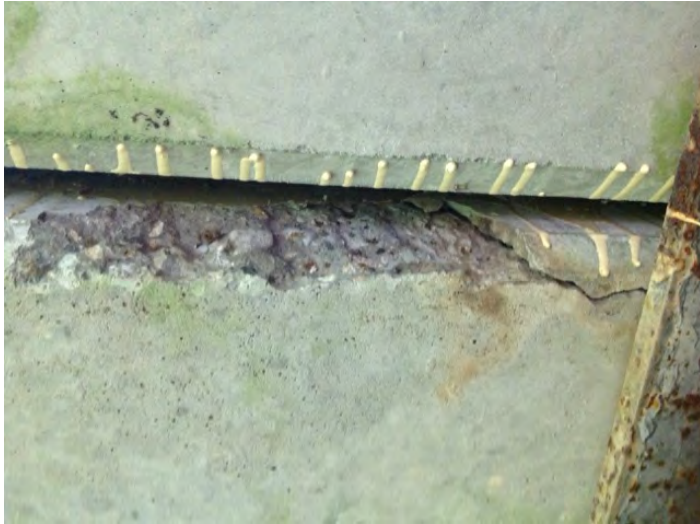
small panel damage
